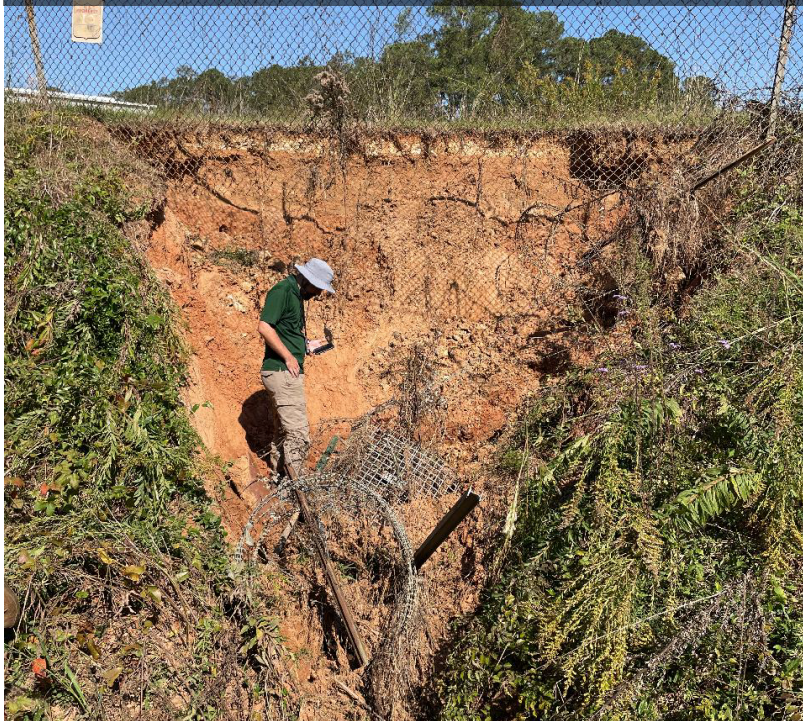
A crew inspects erosion damage to an earthen dam on a retention pond in Edgefield on October 15. Photo by SC Army National Guard on October 15.
