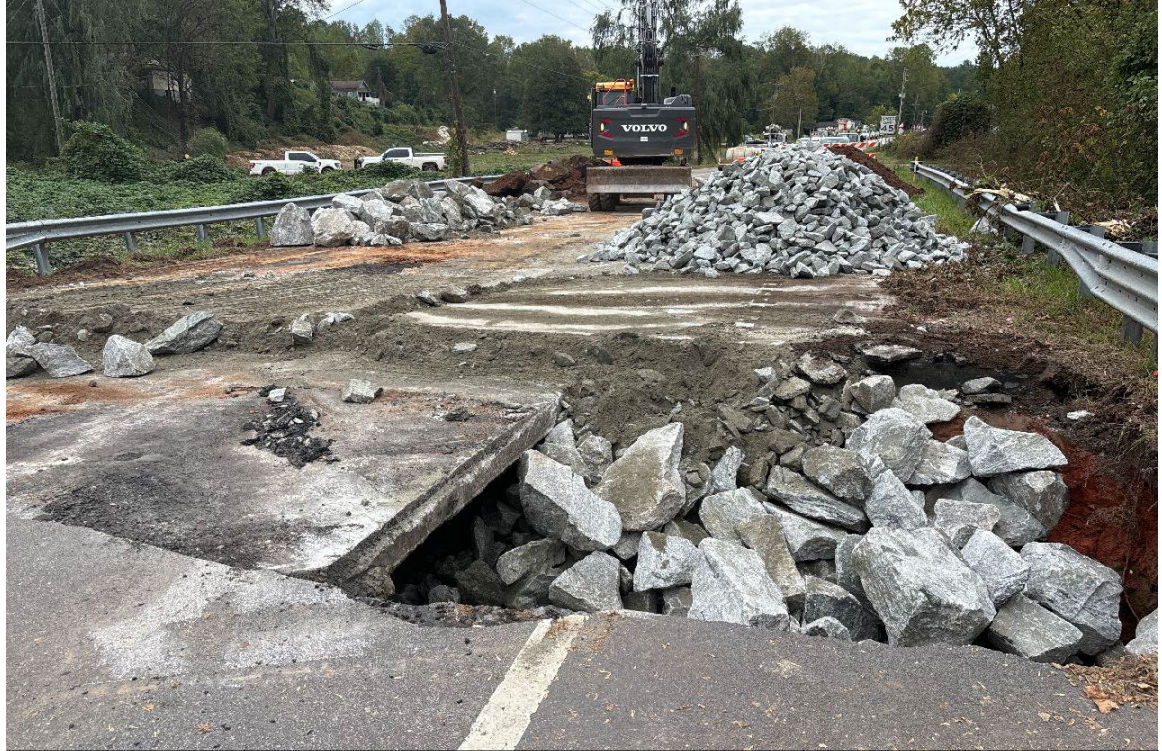
A crew works to repair a washed-out section of U. S. Highway 276 (Geer Highway) just west of Cleveland on October 4. Photo by SC Army National Guard.
