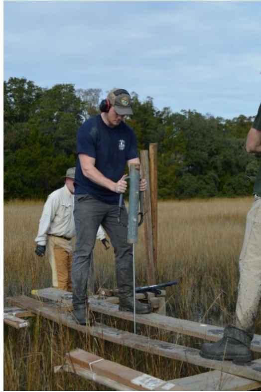
Appendix D, Figure 7. Using a tomato stake driver to drive down first rods.
