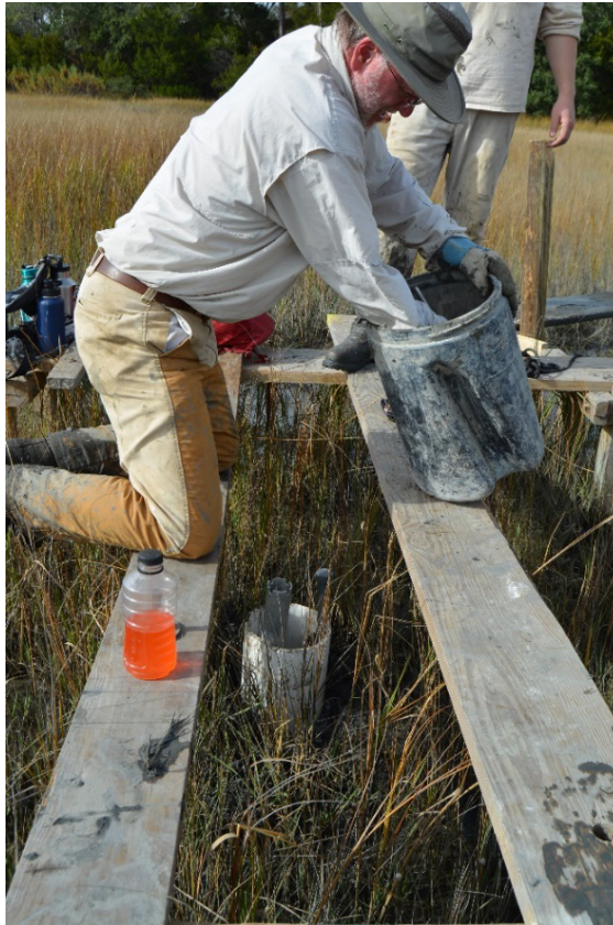
Appendix D, Figure 12. Cement is mixed by hand with water (typically from an adjacent creek, or fresh water brought to the site). The cement is then applied until it is flush with the top of the PVC collar.
