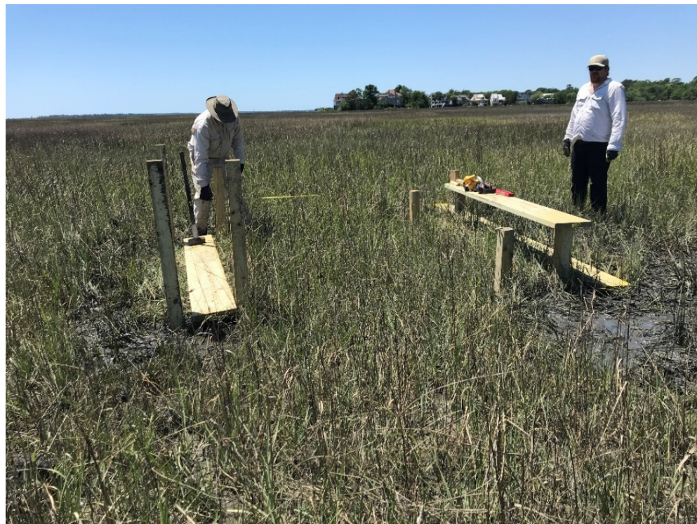
Appendix D, Figure 3. Use a measuring tape to ensure consistent distances between piers. The measuring area should be at least the swing radius of the instrument.
