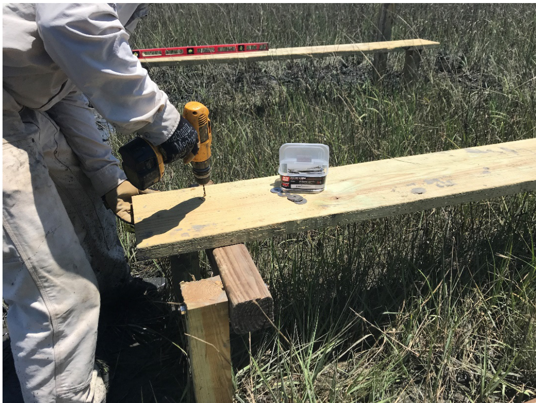
Appendix D, Figure 5. Attach pier boards (2x8's) to the tops of the support boards using screws.
