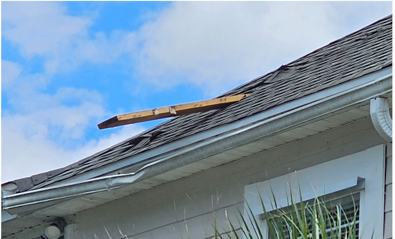
A home along Neptune Street in Edisto Beach had a board driven into its roof by the Second Edisto Beach Debby Tornado.
