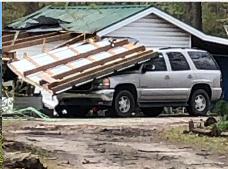
A photo of damage to a home and vehicle along Gunter's Island Road southwest of Aynor in Horry County.
