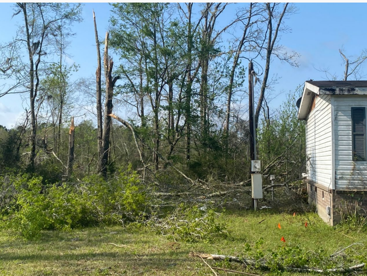
A photo of tree damage and minor roof damage to a home along Bay Road in Marion County.
