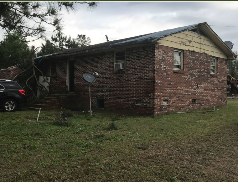
The tornado caused damage to the roof and siding of this home along Greywood Drive in Orangeburg County and dropped a large limb onto it.
