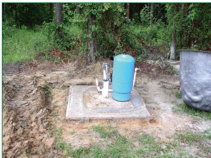
Well & Pumping Plant ~ Bryan Farms
